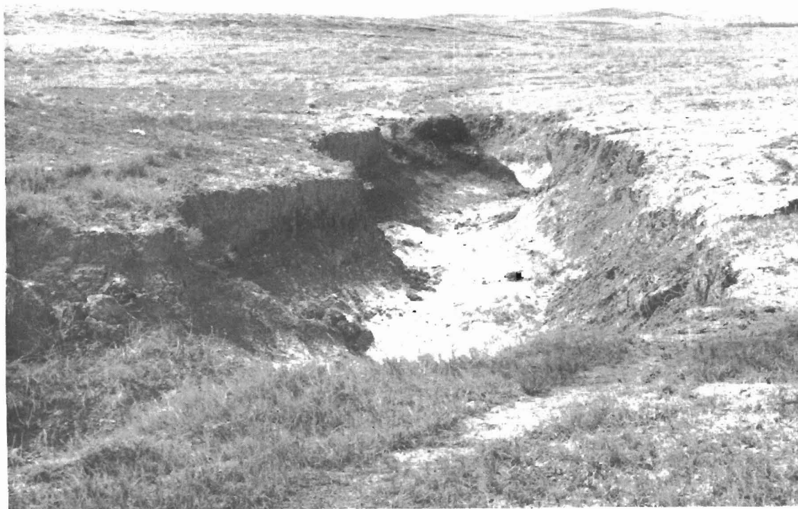
Figure 2. Gully forming in area where the cover of grass is thin. Photo by Bob Runner.
