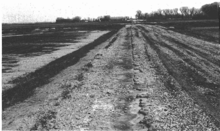
Figure 7. Damage to rural roads south of Grand Forks. A small bridge at the northeast corner of a section was washed out when floodwater breached the road surface. The lower photo shows how the gravel has been washed off the road into the ditch north of the road.
