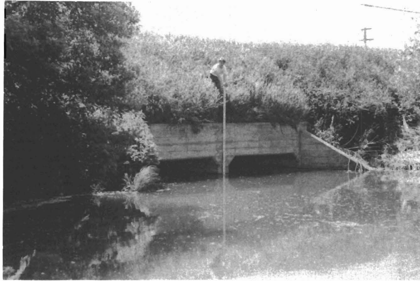
Figure 47. Culverts beneath the Burlington Northern Railroad tracks at the south edge of the University of North Dakota campus. Each culvert has a cross-sectional end area of 130 square feet (6.5x10 feet). A culvert system this size can handle a maximum flow of approximately 1,875 cu ft/sec before water starts backing up.
