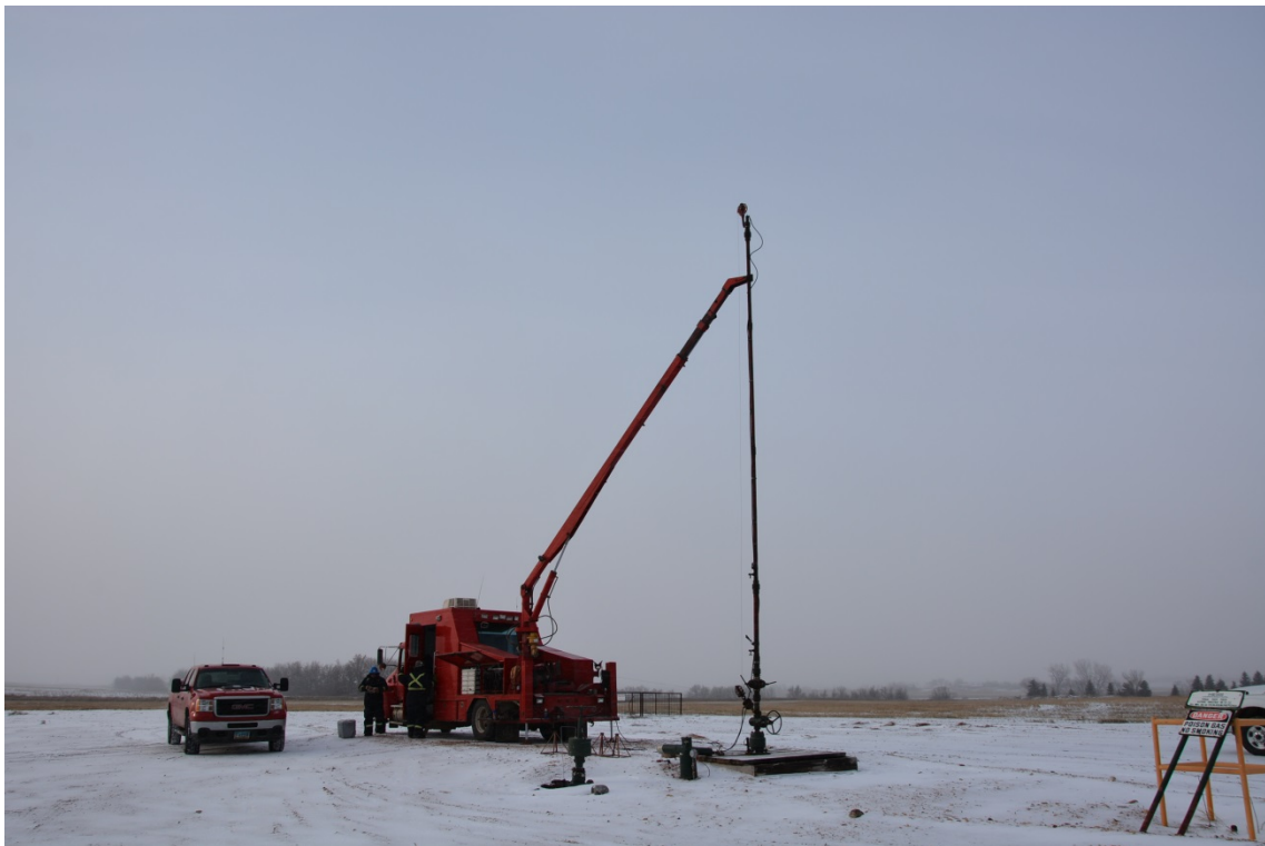
Figure 3. Slickline unit set up over NDIC Well # 12363, Astrid Ongstad 14-22 north of Tioga, ND.
