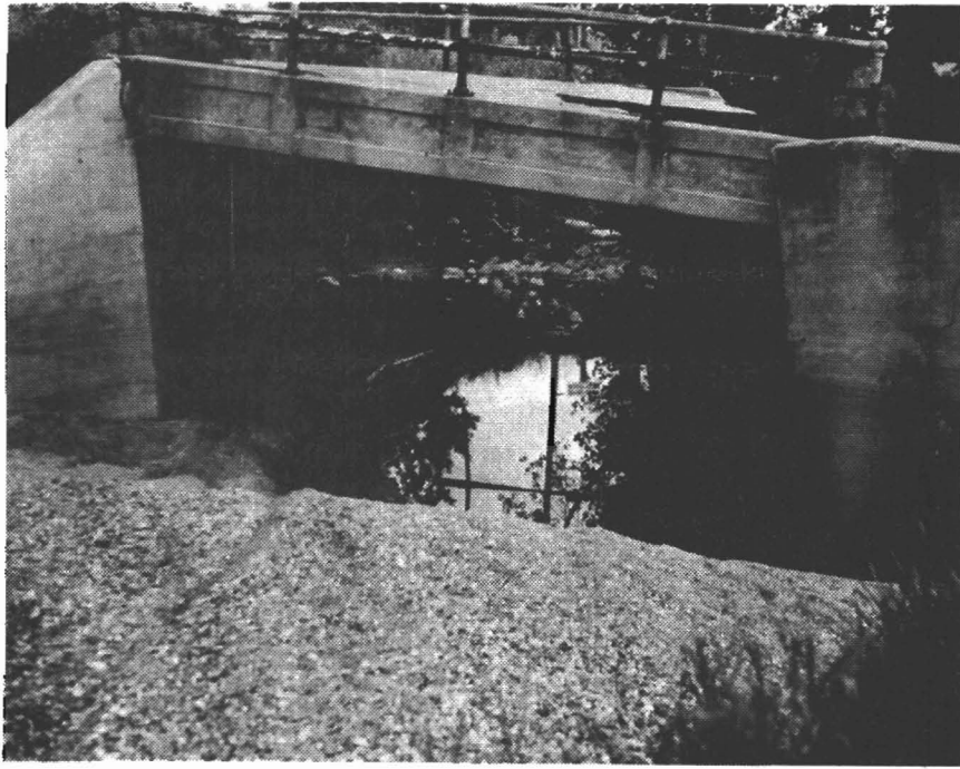
Figure 8. Damage to bridge crossing Second Larson Coulee by flooding. Location: NE \frac{1}{4} NE \frac{1}{4} sec 5, T154N, R82W.
